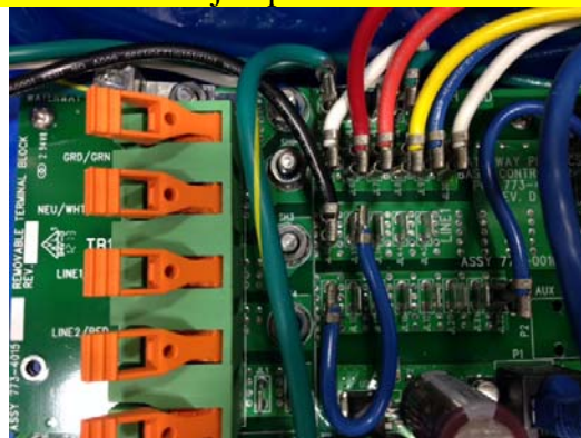
↖ Blue Jumper wire between JL13 & JL15
